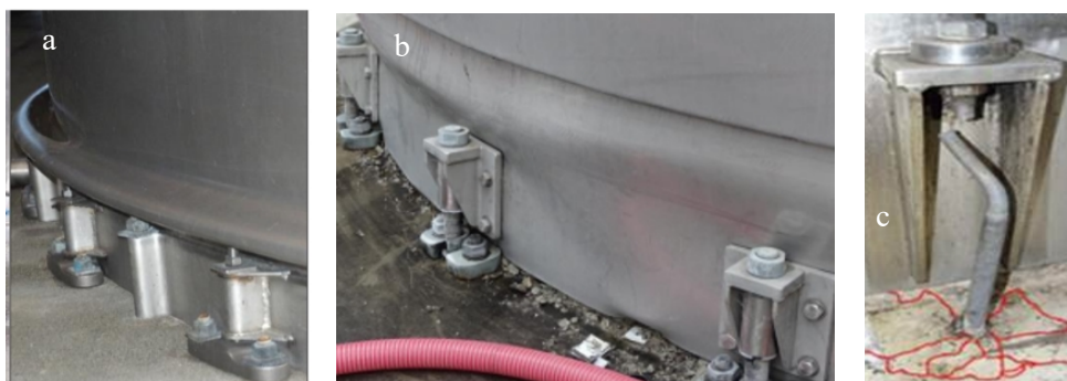
Figure 2: Reported damage in Kaikoura earthquake; (a, b) Barrel buckling; (c) Rod rupturing [12]
