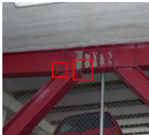
Figure 3. Fracture in EBF Link due to inadequate load-path (Clifton et al., 2011)
