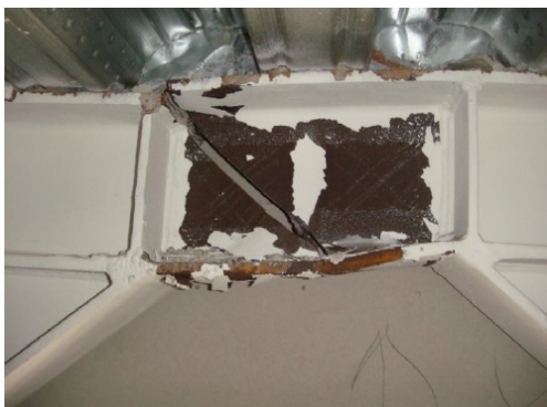
Figure 1. Fractured EBF link in Pacific Residential Building (Clifton, Bruneau, MacRae, Leon, & Fussell, 2011)
