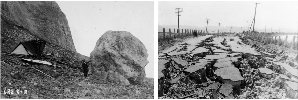
Figure 2: Geotechnical failures in the 1931 Napier earthquake L: landslide, R: Liquefaction lateral spread
