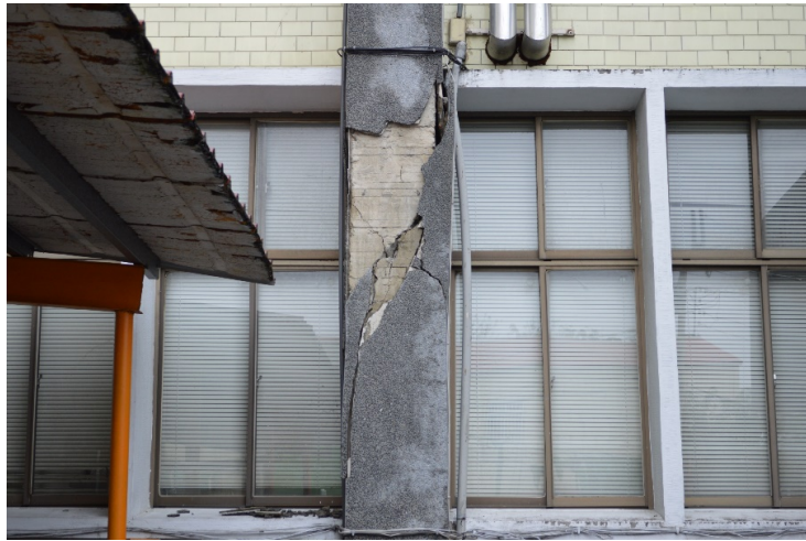
Figure 3: An example of structural damage classified as severe by Laughery et al. (2020).
