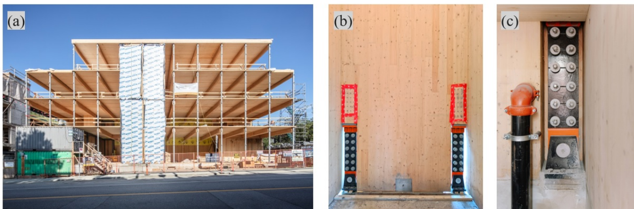
Figure 9: (a) full building elevation (b) CLT wall base (c) installed seismic devices
