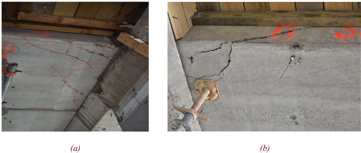
Figure 4: Examples of beta units damage observed a) previously unidentified damage pattern b) transverse cracking at the unit soffit accompanied by longitudinal cracking
