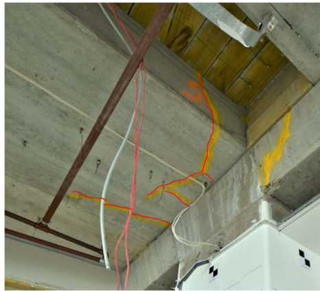
Figure 5: Damage sustained in hollow-core unit under low drift levels
