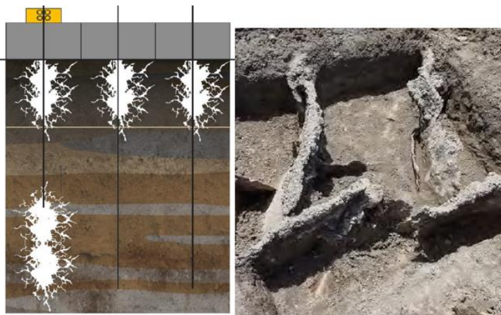
Figure 5. Mainmark’s resin injection process (left) and hand-exhumed resin veins (right), after Traylen et al (2017)
