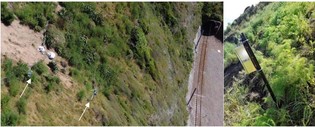
Figure 4: Monitored catch fences (arrowed) at NIMT 33.44; tilted sensor at right after movement
