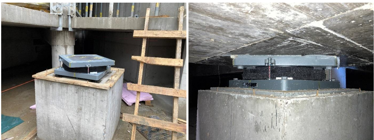
Figure 9: SIP®-V devices within BioSense Research Institute; during installation (left) and installed (right)
