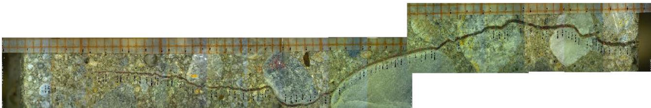
Figure 3: Image of a structural crack in reinforced concrete from the experiments of Borosnyói and Snóbli (2010); Note: the surface of the concrete member is at the right side of the image and the level of the reinforcing bar is at the left side of the image (Borosnyoi-Crawley and Gyurkó-Nagy, 2023).
